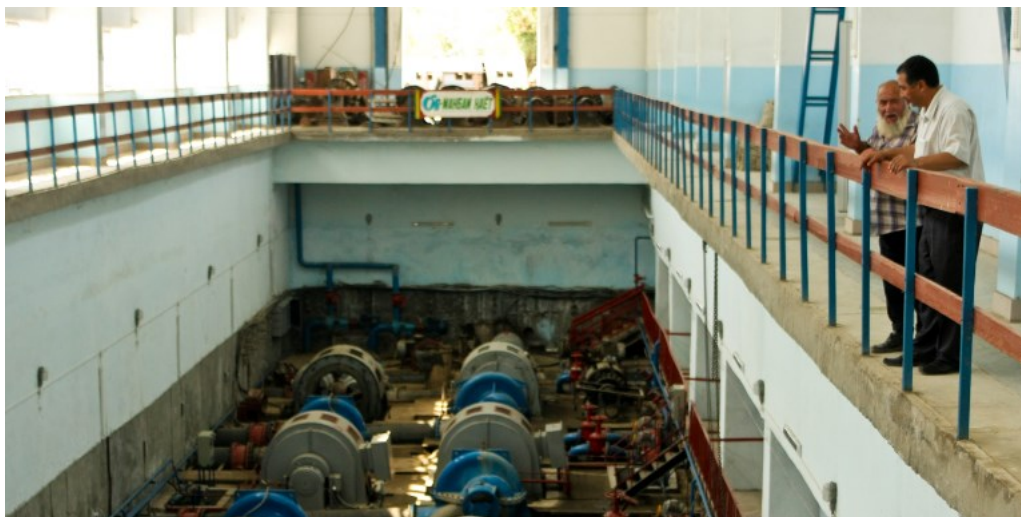
A view of a water pumping station in Tajikistan. Photo Credit: ADB.
