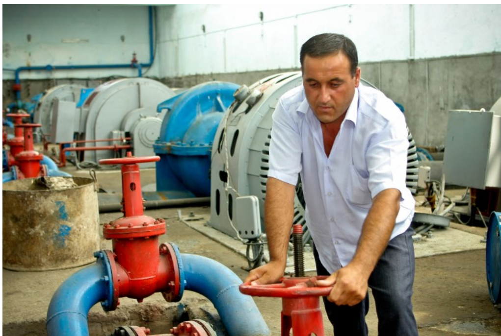
A man working at a water pump station in the Asht District in Tajikistan. Photo Credit: ADB.
