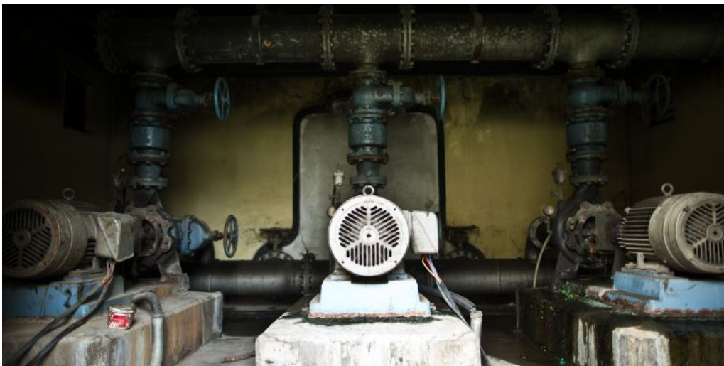
Water pumps in a village in Nepal. Photo credit: ADB.
